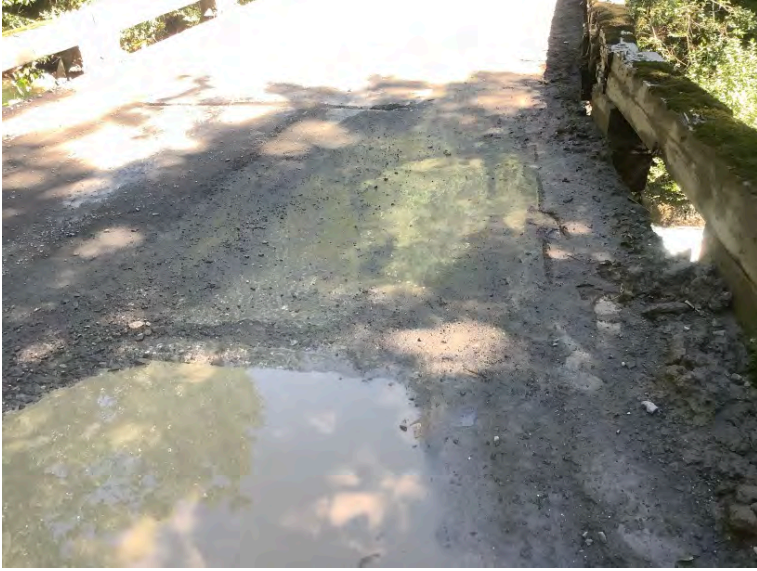
Approach pothole with ballast wall wear
